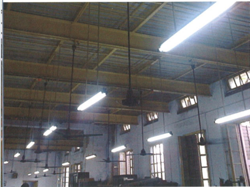
The damaged ceiling of Physics Laboratory
